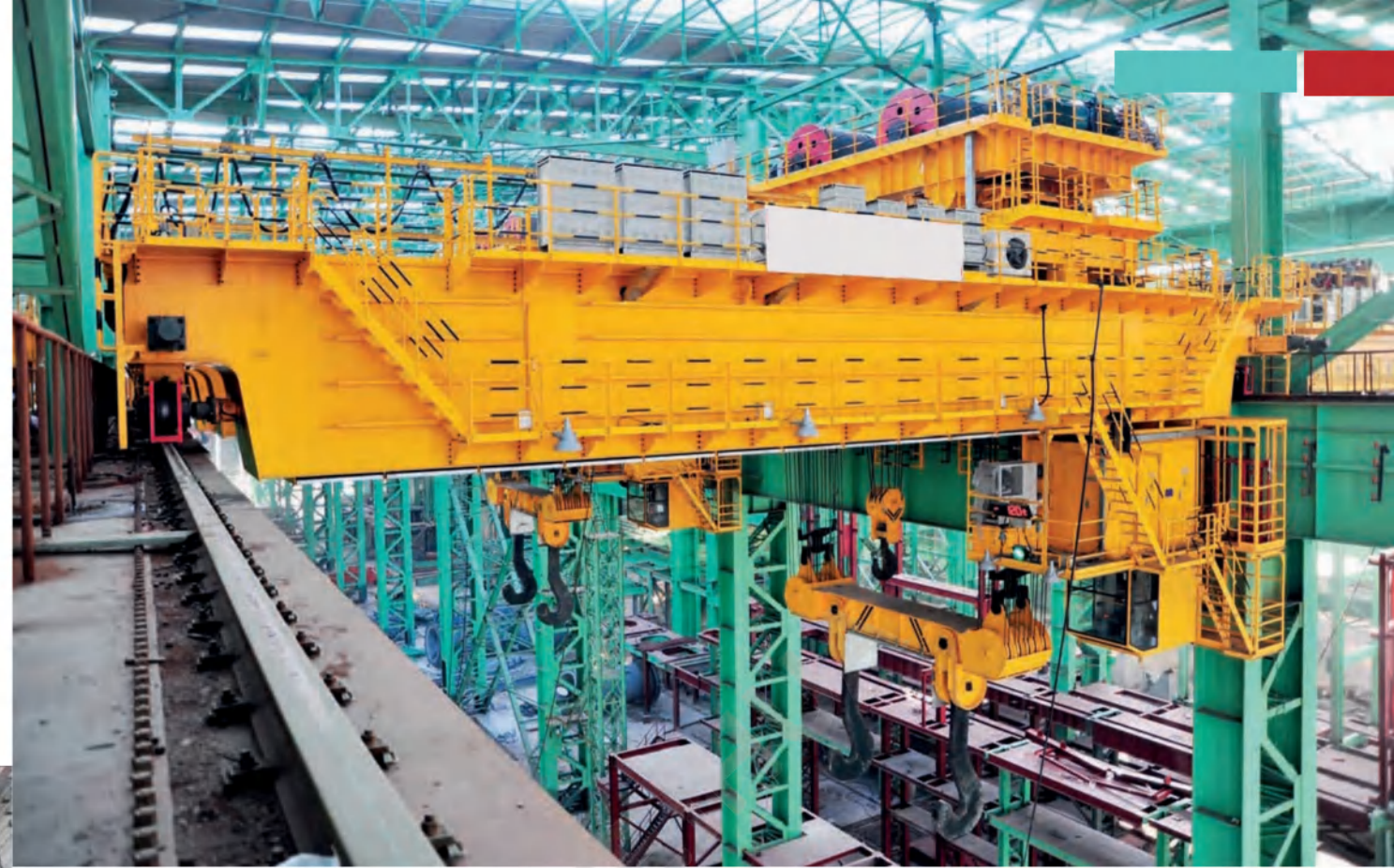
320吨四梁六轨铸造起重机 320t ladle crane with four girder and six rails
