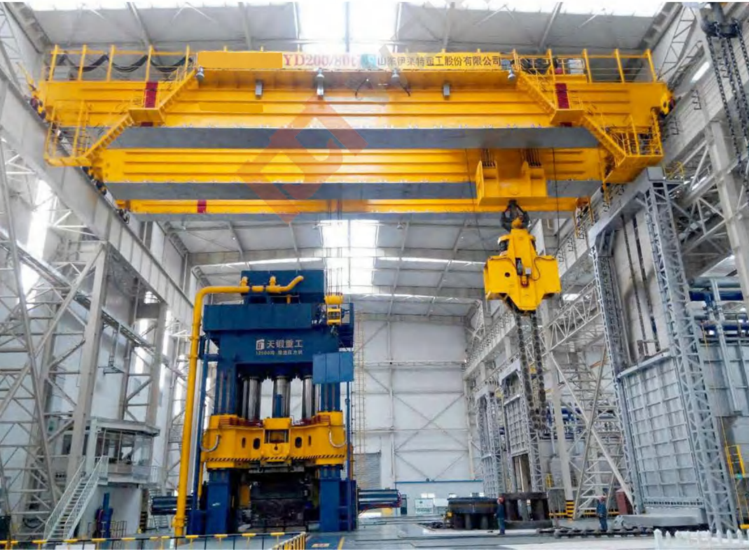
▼ 250t锻造起重机 250t forging crane
